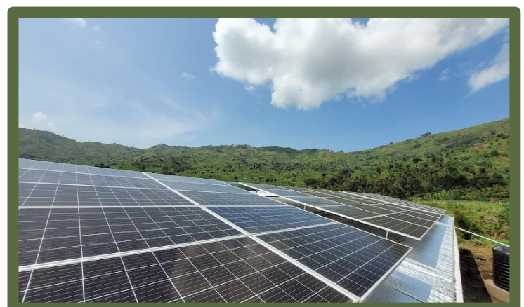
Solar panels sourced from an East African partner, African Energies, on the roof of Mbata Smart Agri-Centre.
