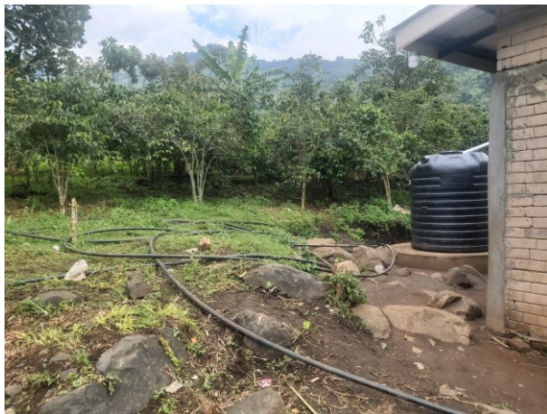
Water supply installed at the FEC
